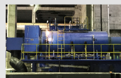
Heat Recovery System
